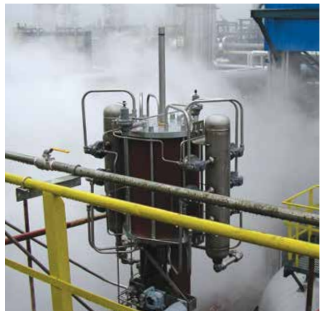
SVI II AP on steam conditioning valve
